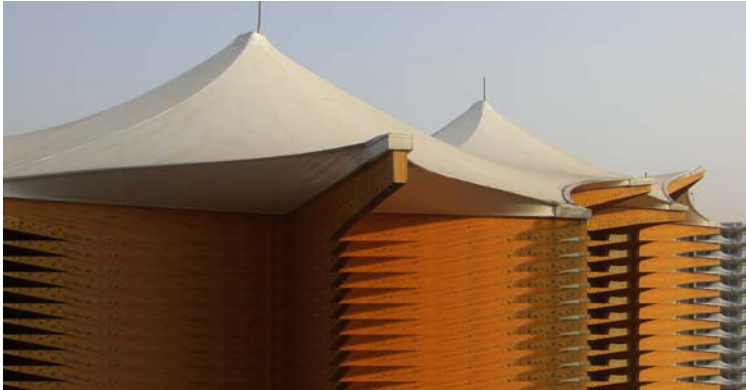
Fig. 7: The roof of the Norwegian pavilion at 2010 EXPO, Shanghai: Application of URS.
